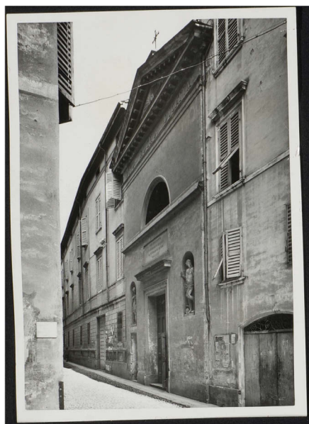
Fig. 2.1. The demolition of the Church of San Rocco in Cavallerini street (external view), 1951. By permission: Biblioteca civica d'arte Luigi Poletti — Modena (Italy).
